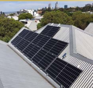
3.2 kW of REC N-Peak in Perth, Australia; world's first installation using REC N-Peak panels
